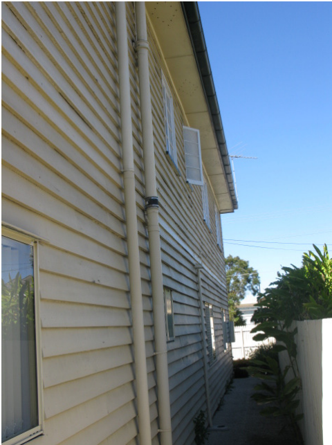
Picture 3 - external photo of the side wall on western side - the bathroom windows can be seen above the lounge room ceiling area where the damage is.
