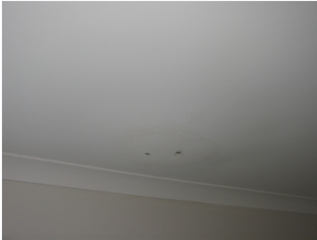
Picture 1 - ceiling of downstairs lounge room
